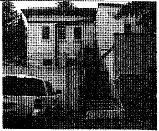
Stairs allow access to lower roof and anyone has access to the below pictured area
